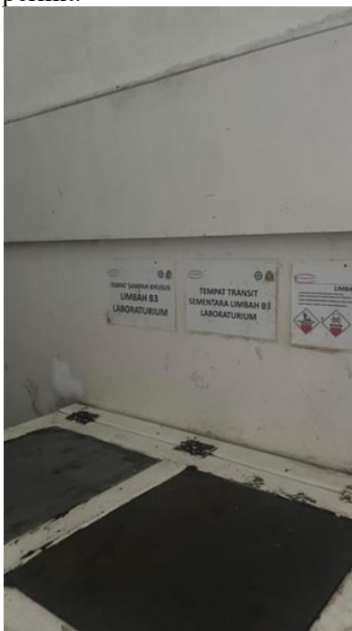
Figure 1 Temporary Storage Area for B3 Waste at PT NICO Source: Research Documentation, 2026.
