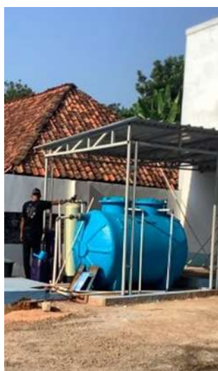
Figure 2 Wastewater Treatment Plant (IPAL) SPPG Cijunti
